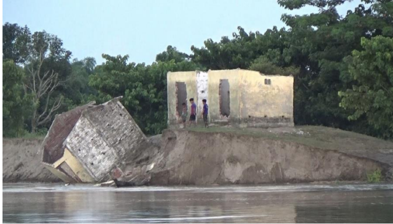
A primary school breaking away in Majuli due to river erosion (photo credit: Mitu Khatanar)
