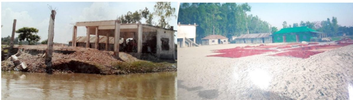
Washed away school building in Shapdhuri Union
